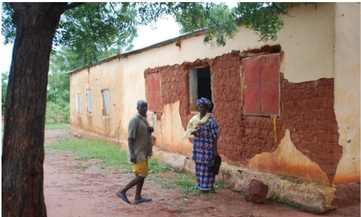
The village school in Pimperna which has been constructed by the population itself is in bad shape: improving the number and quality of the classrooms as well as the are among the community’s priorities.
