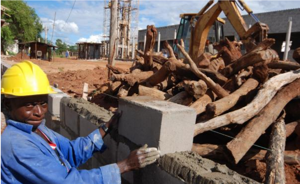
In Namapa the ministry of health renovates and expands the rural hospital.
