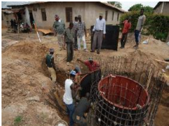
Switzerland supports the water authorities of the city of Dodoma in their effort to enlarge its disposal network in the different neighbourhoods.
